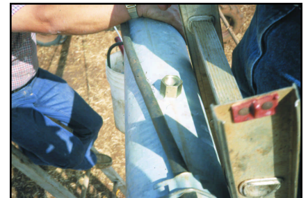
Figure 14. Swedge coupler installed.
